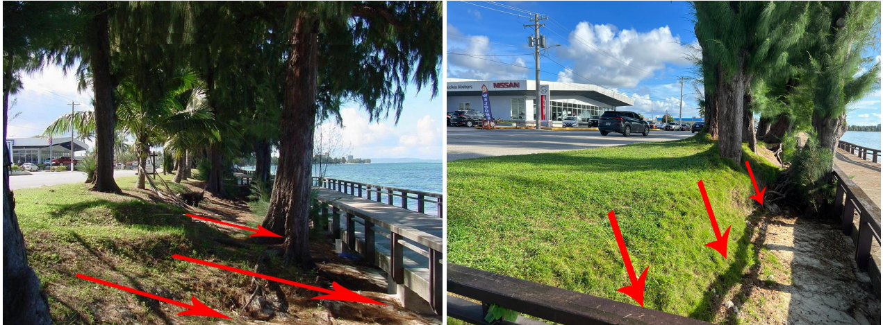
FIGURE 2: (Left) Beach Road, prior to Typhoon Yutu in 2015 and (Right) Beach Road Today, October, 2022. The effects of Typhoon Yutu, Typhoon Soudelor, and many more tropical depressions have caused the face of Beach Road to drastically change. The first change is a decrease in the number of trees that act as a natural support structure of the coastline. The second is a significant change in the berm due to sediment loss. (Left Picture Credit: U.S. Army Corps of Engineers)
