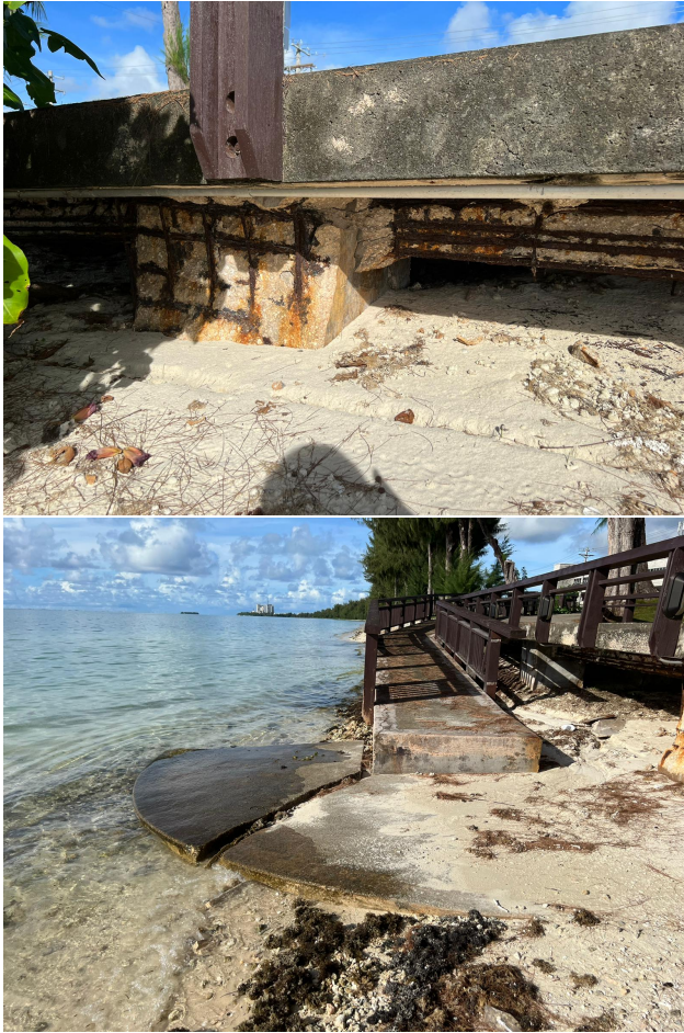
FIGURE 4: The upper picture showcases the power of waves as one can observe exposed concrete reinforcing bars. In the lower picture we can observe collapsed or missing sections of an accessibility ramp from the walkway to the beach. These observations were the basis for testing our inclined wall seawall as there is potential for the water facing beams to collapse. This would then act as an inclined ramp for waves to travel over and onto Beach Road. Pictures taken in summer 2022.
