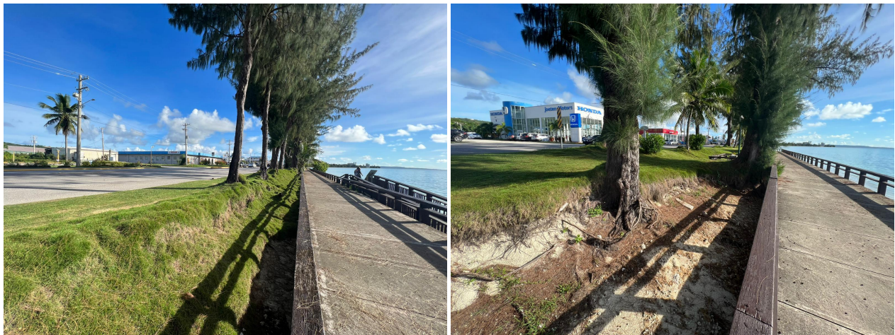
FIGURE 3: Beach Road and the pathway that runs parallel to it. In the right picture we can readily observe how waves have eroded away sediment such that tree roots have become exposed. Further, notice that waves have caused a vertical drop to develop. The exposed tree roots indicate that this “buffer zone” was covered with soil, but a constant barrage of waves and storms has altered Saipan’s coastline. It is important to note that waves do not normally reach this buffer zone under normal tidal fluctuations. Instead, this erosion indicates that waves now have enough energy to traverse Saipan’s barrier reef and reach the buffer zone of Beach Road.
